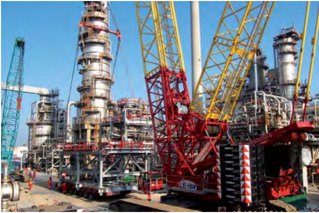
Light Cat Naphtha pre-assembled unit arrived at the site during construction of Sriracha Clean Fuels Project.
