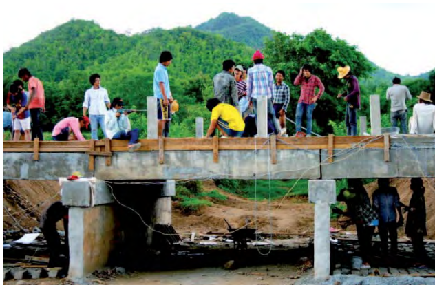
Chulalongkorn University engineering students applied their engineering knowledge in building public amenities in remote areas.
