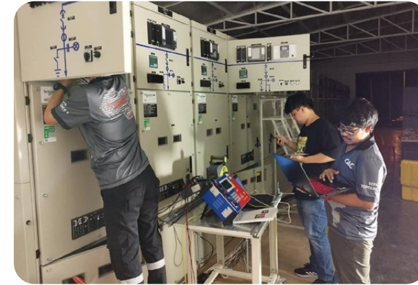
Picture depicts Testing and Commissioning work at Tha Yang substation, Phetchaburi Province
