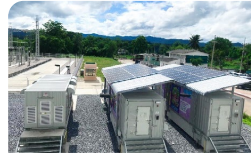
Picture depicts Battery Energy Storage System, size 3 megawatts / 2.2 MWh of Microgrid Development Project at Mae Sariang District, Mae Hong Son Province Project of the Provincial Electricity Authority.
