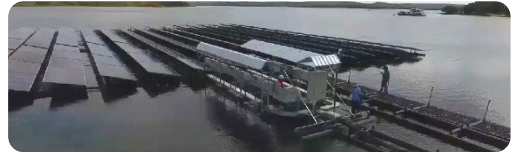
Picture shows the floating solar farm project at Sirindhorn Dam, size 256 kilowatts
