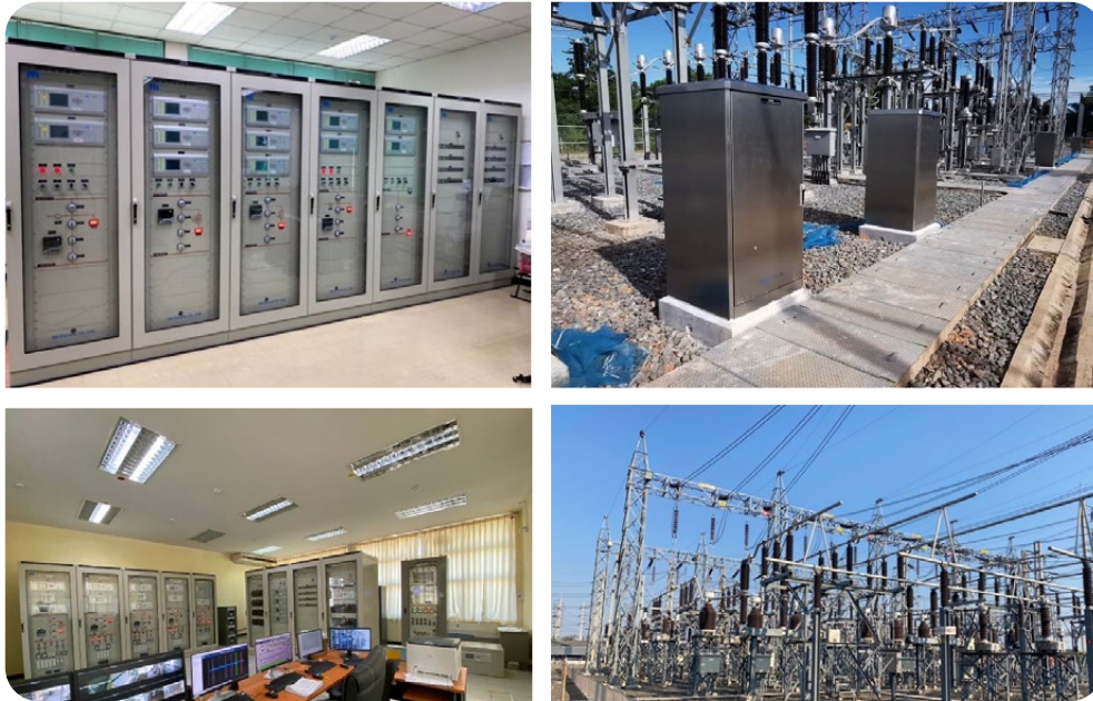
Picture depicts the installation of substation control and protection system according to IEC61850 technology
