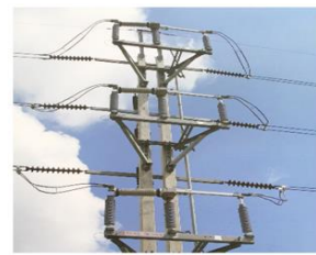
69, 115kV Load Break Switch
