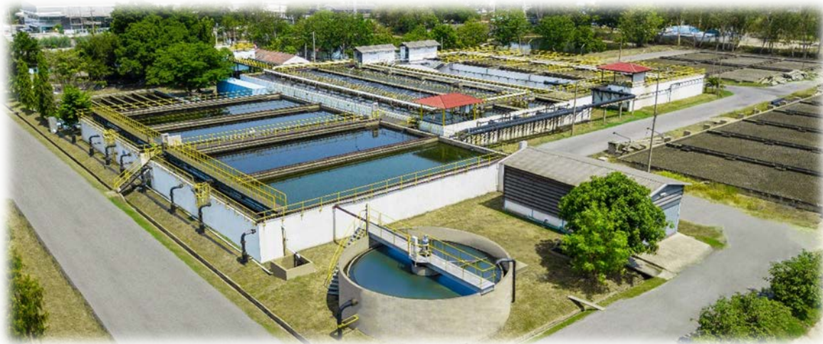
Water Production and Wastewater Treatment Projects, Bang Pa-in Industrial Estate
