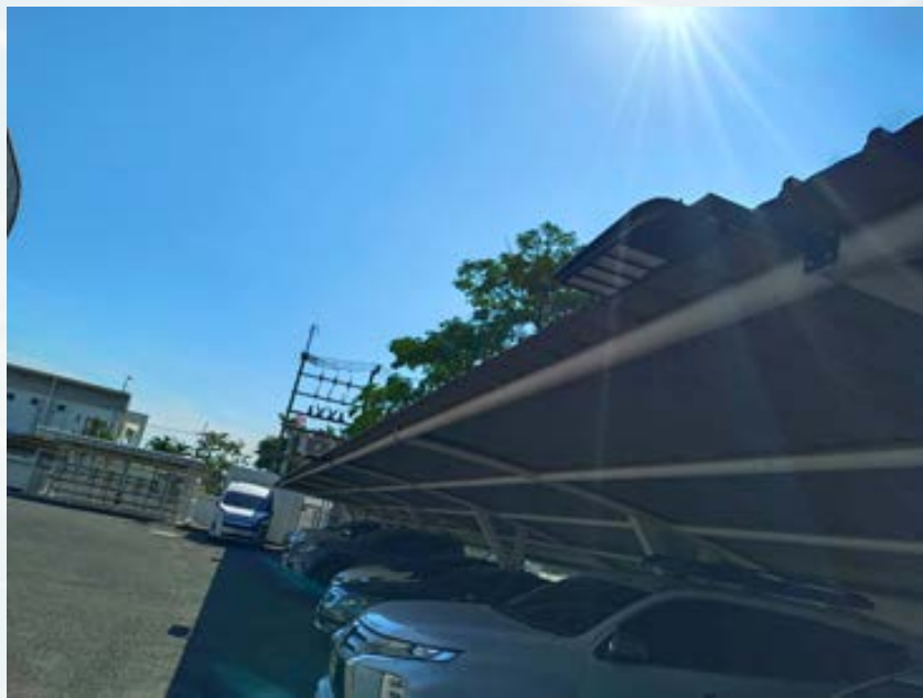
Solar Panels Installed at Parking Lots
