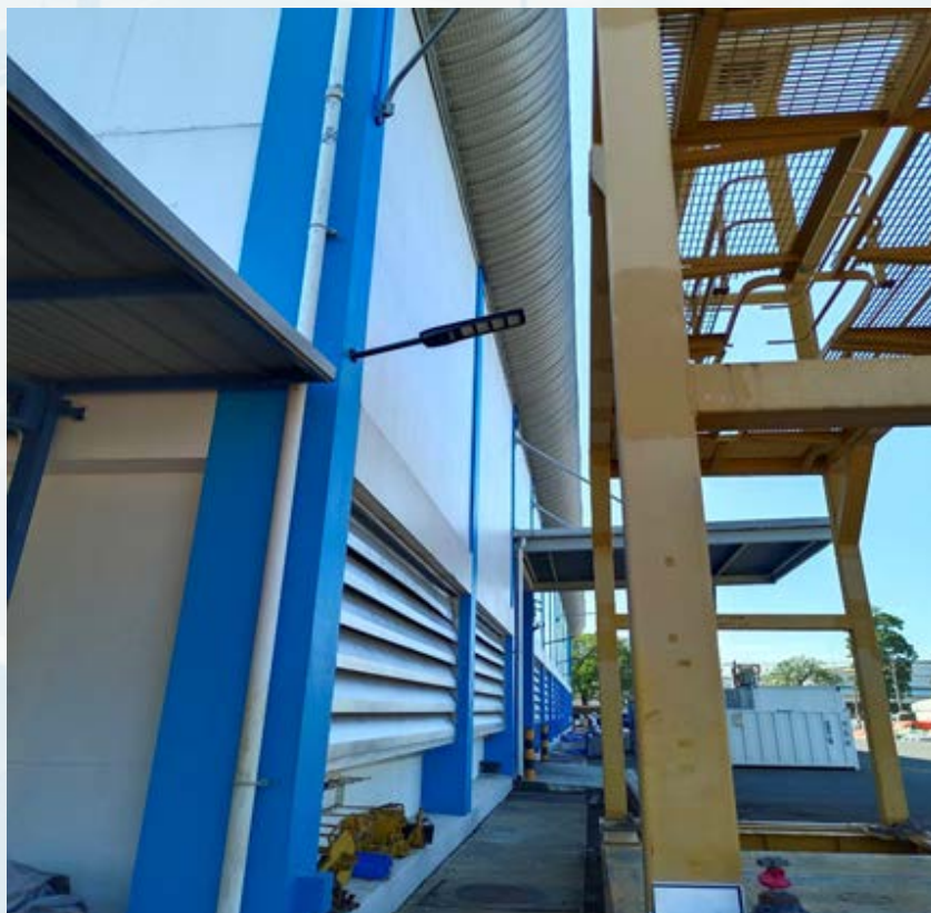
Solar Panels at Building Trims
