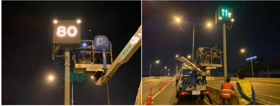
Notification of lane closure and display of recommended speed via the Matrix Sign
